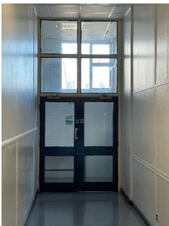
Figure 17 The evacuation wayfinding signage hidden by the cross-corridor door
