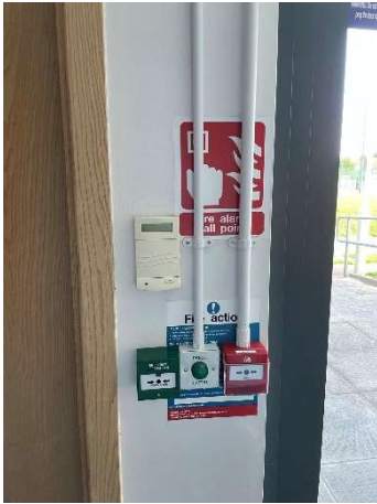
Figure 13 An example of where equipment has been installed on top of signage
