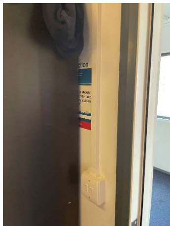
Figure 27 An example of an evacuation sign covered by a cupboard so it can't be read
