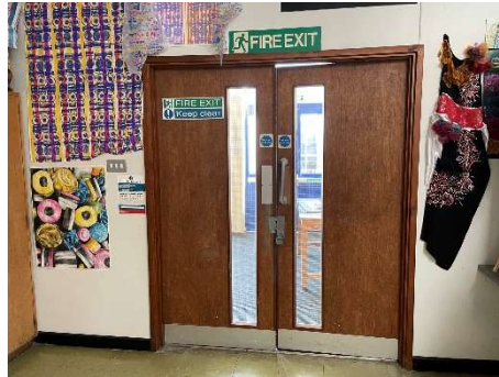
Figure 20 An example of a fire door not closing properly
