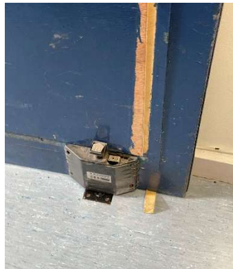
Figure 04 An example of a Dorgard with a flat battery propped with a wedge
