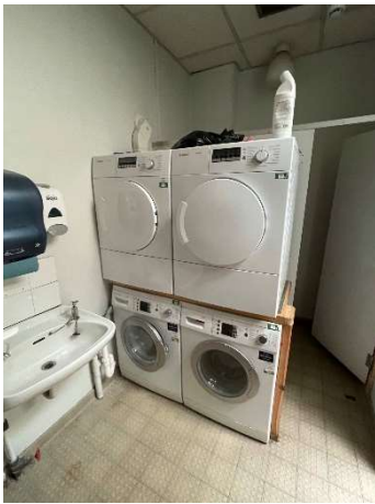
Figure 15 The PE washing machines and tumble dryers that must be correctly managed
