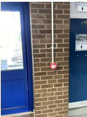
Figure 11 An example of where signage has never been installed
