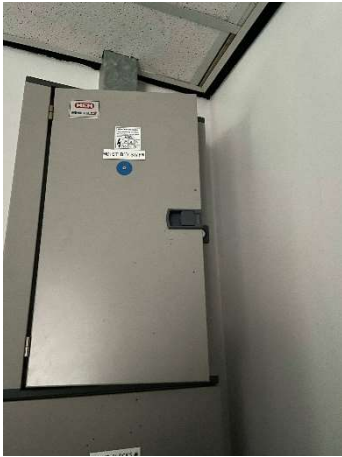
Figure 07 An example of a distribution board found open
