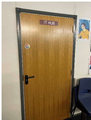
Figure 25 An example of one of the fire door symbols covered by a sticker
