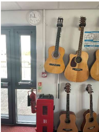
Figure 23 The musical instruments in the way of the fire equipment
