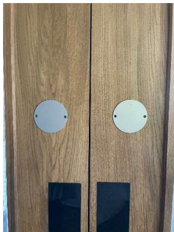
Figure 26 An example of where fire door signage must be replaced as it can no longer be read
