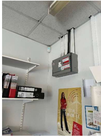
Figure 08 Another example of a distribution board found open
