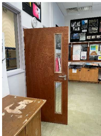
Figure 18 An example of a newly installed fire door with no closer or signage
